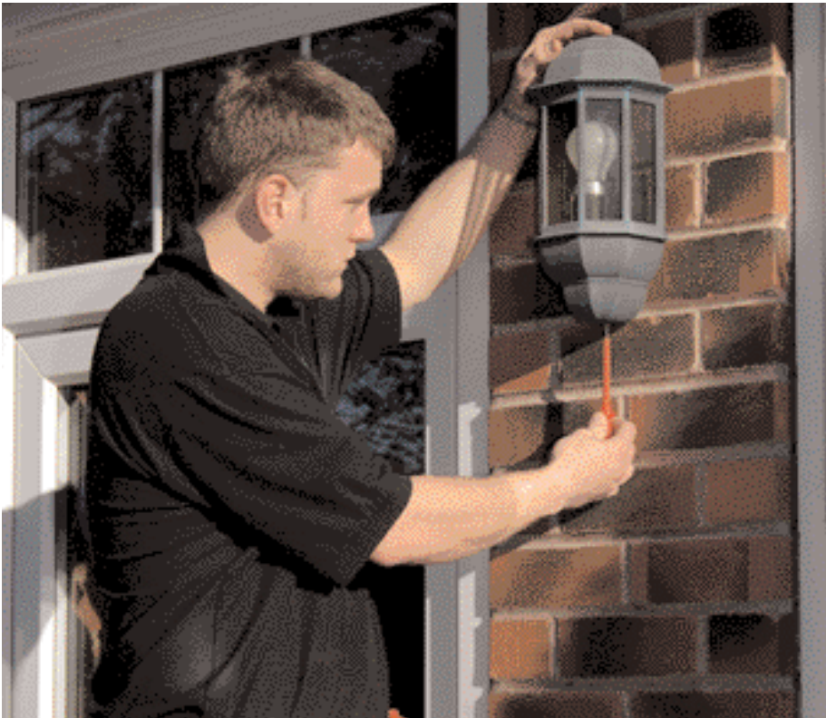
Outside Lighting subject to Part P
