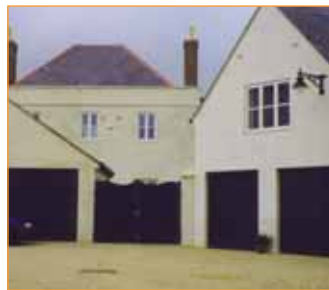
A much less successful courtyard: overlooking is minimal and series of garage doors and gates is forbidding.
